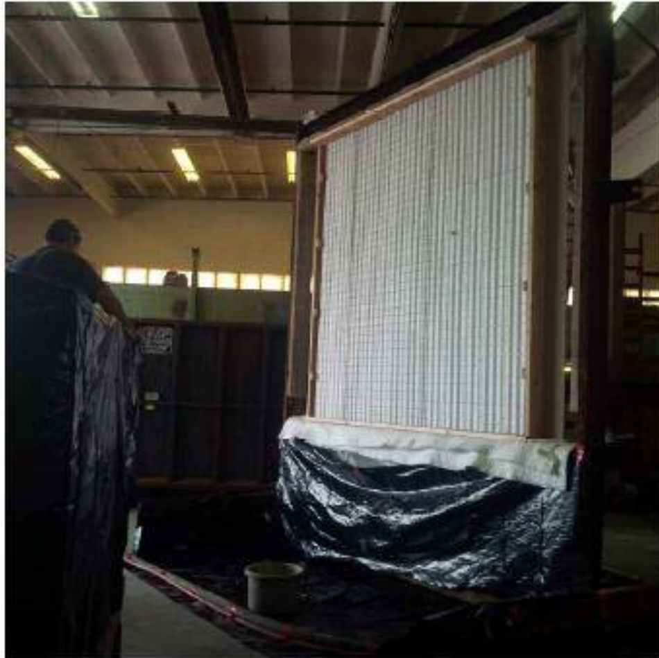
Photo 6 Schnell Wire Systems s.r.l. Wall Sample Installed in Test Fixture Prior to Concrete Application
